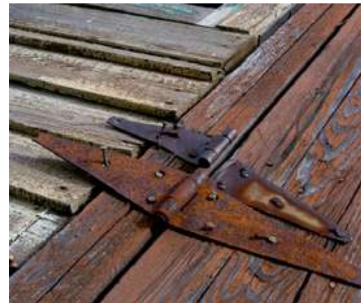
Rusty hinges on a building exterior Source Wikipedia
