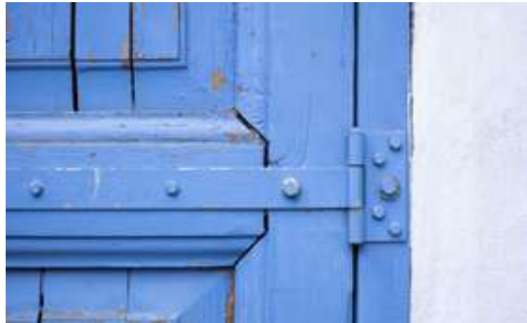
Close-up of a weathered blue wooden door featuring rusty hinges and peeling paint. Source : Pexels
